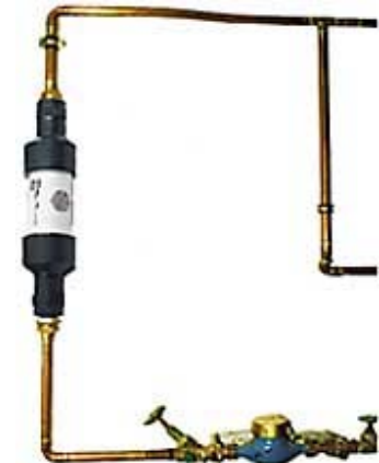
Installation in the tap water pipe after water meter
